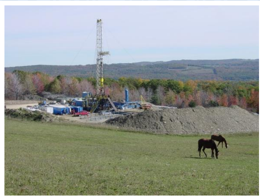
Photo courtesy of the NYSDEC field inspection team.
